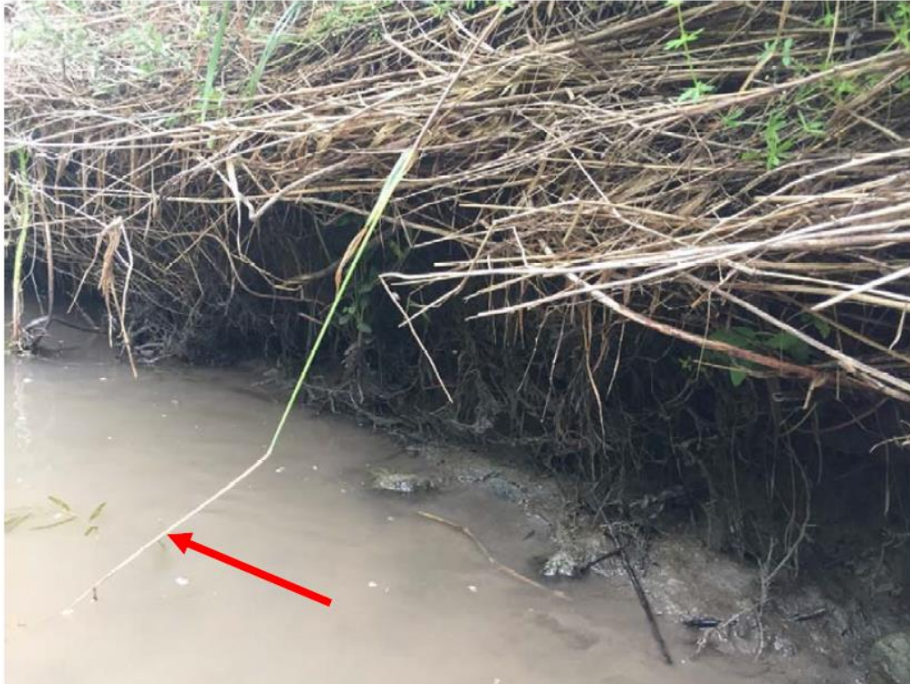
Figure 1-1 Undercut bank along EB3
