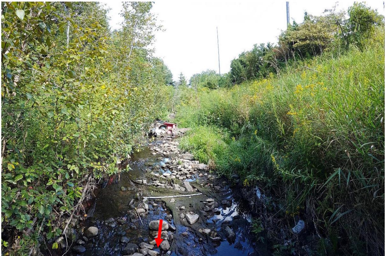
Figure 1-2 Exposed Non-woven Geotextile on Bed at WB6
