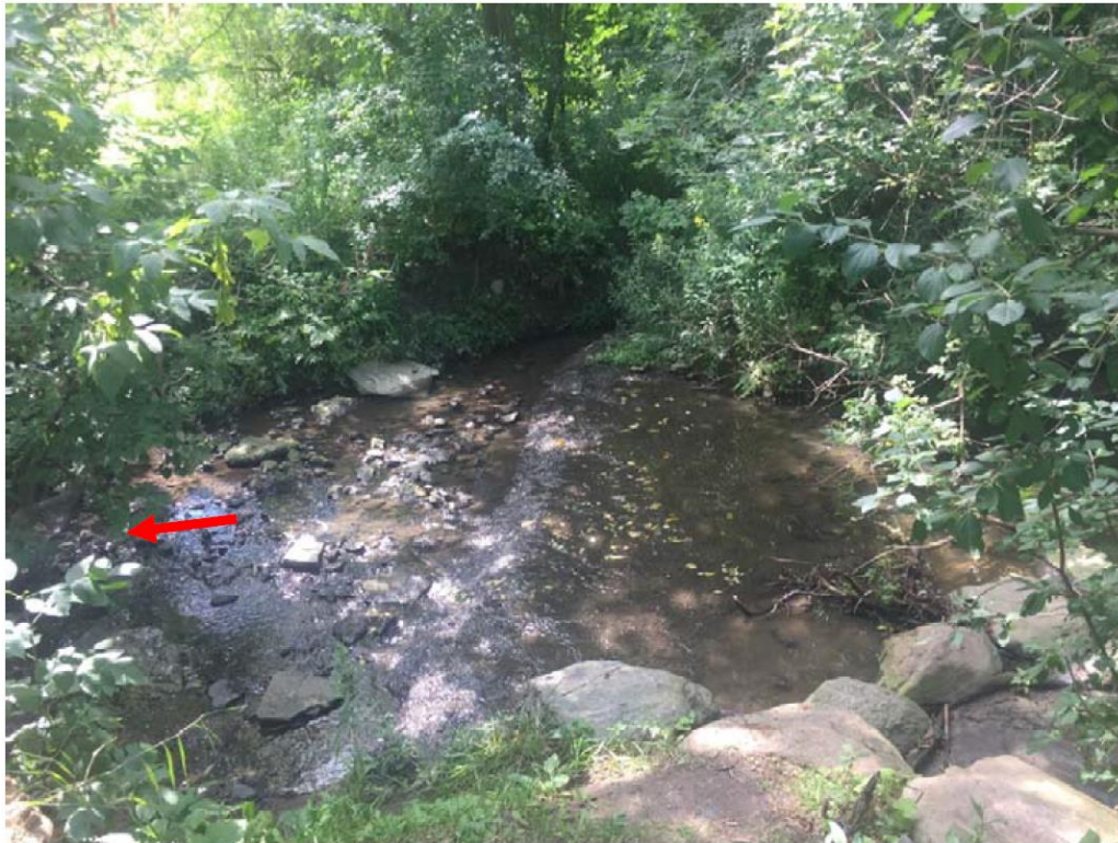
Figure 1-1 Possible Exposed Concrete Pipe at EB7
